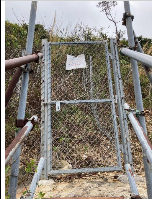
Photo 2 – Current situation of fencing and warning sign
